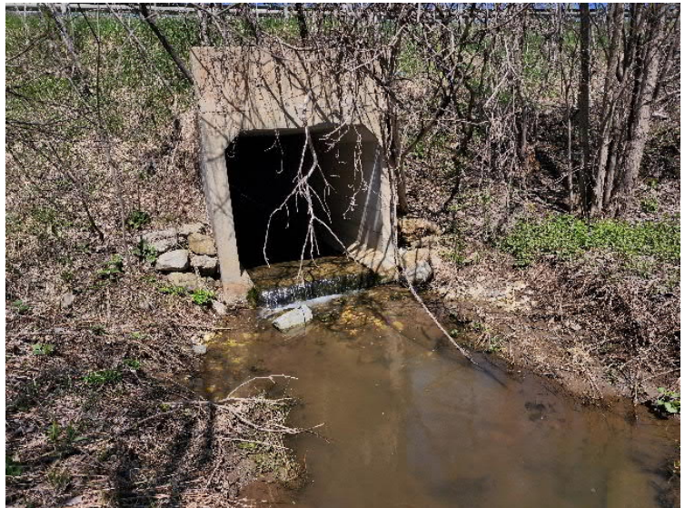
Photograph 2. South side of box culvert under Sperry Road and stream. View looking north.
